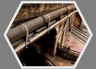
OVER 20,000 MILES OF PIPES
